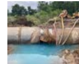
Water Main Breaks
